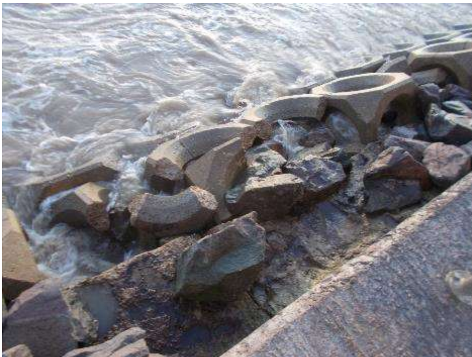
Figure 4-13: Failed blocks near east end of concrete block revetment
