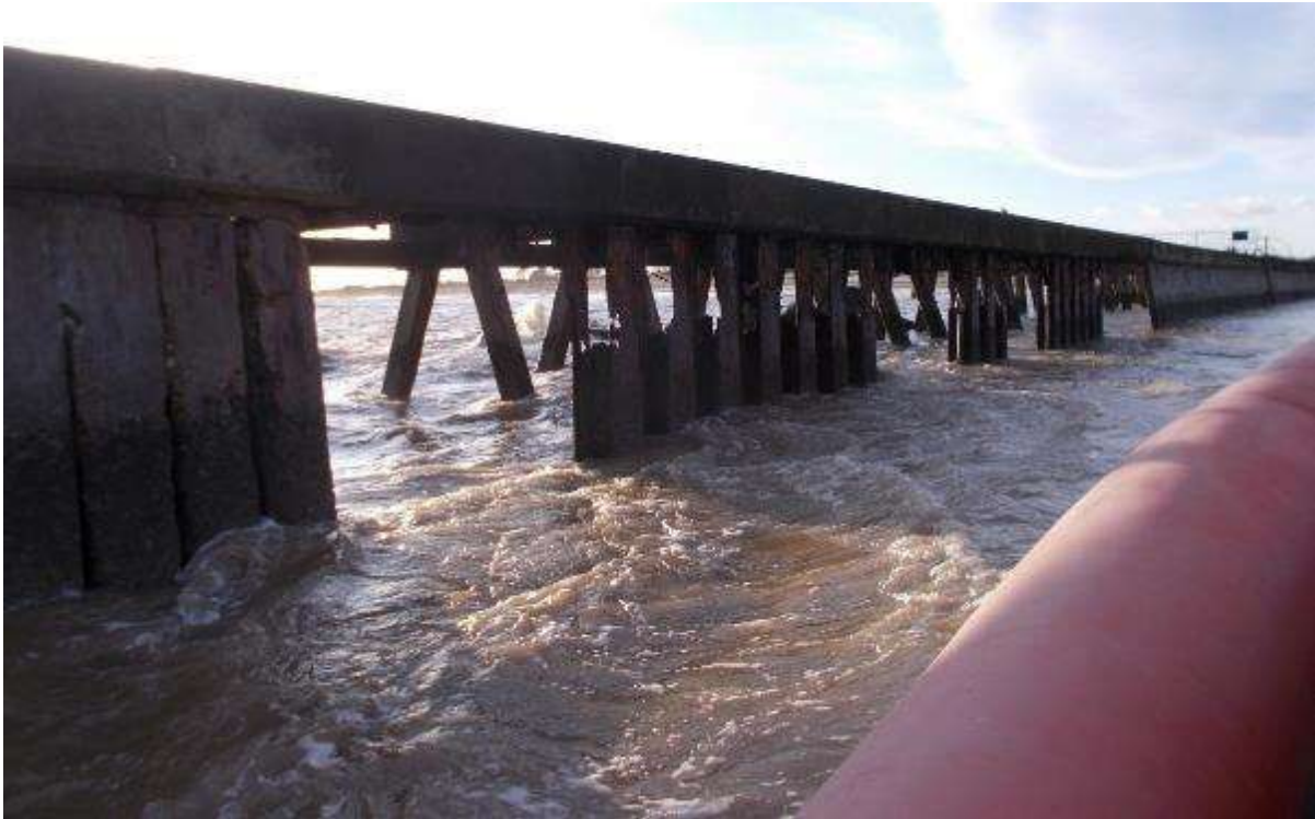
Figure 4-5: Length C corroded steel sheet piles and unsupported front beam.
