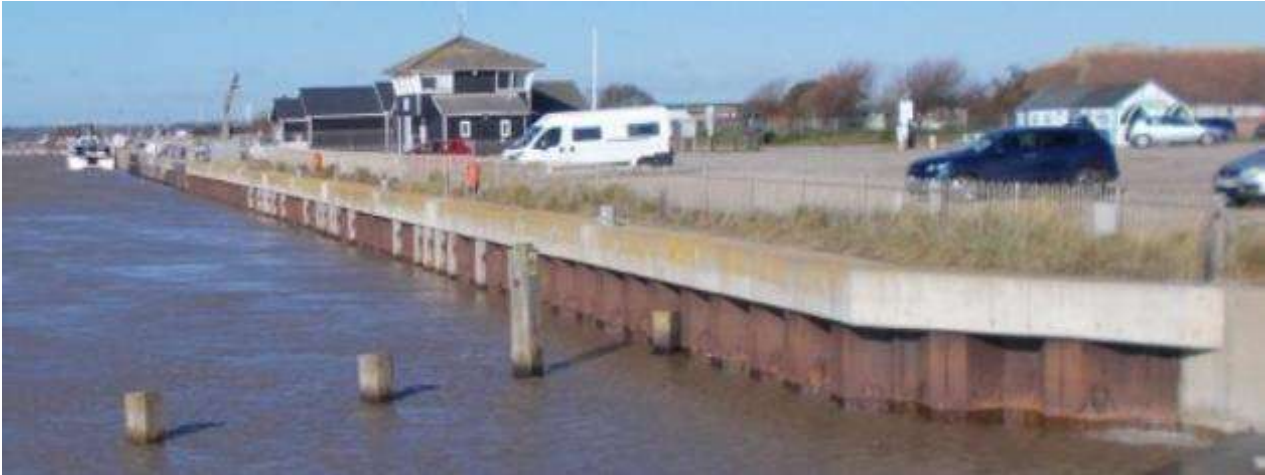
Figure 4-18: Current condition of North Wall
