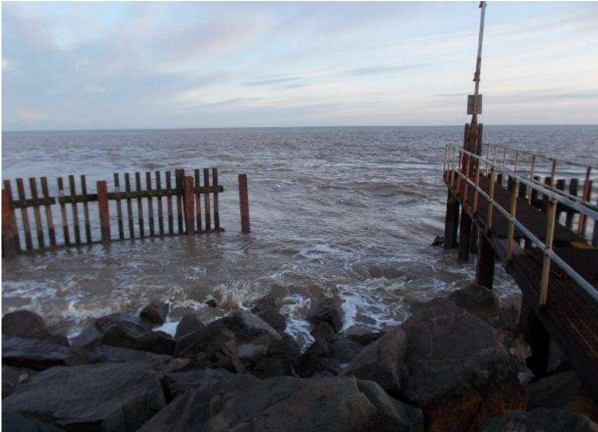
Figure 4-14: Rock armour, navigational light and damaged timber fendering
