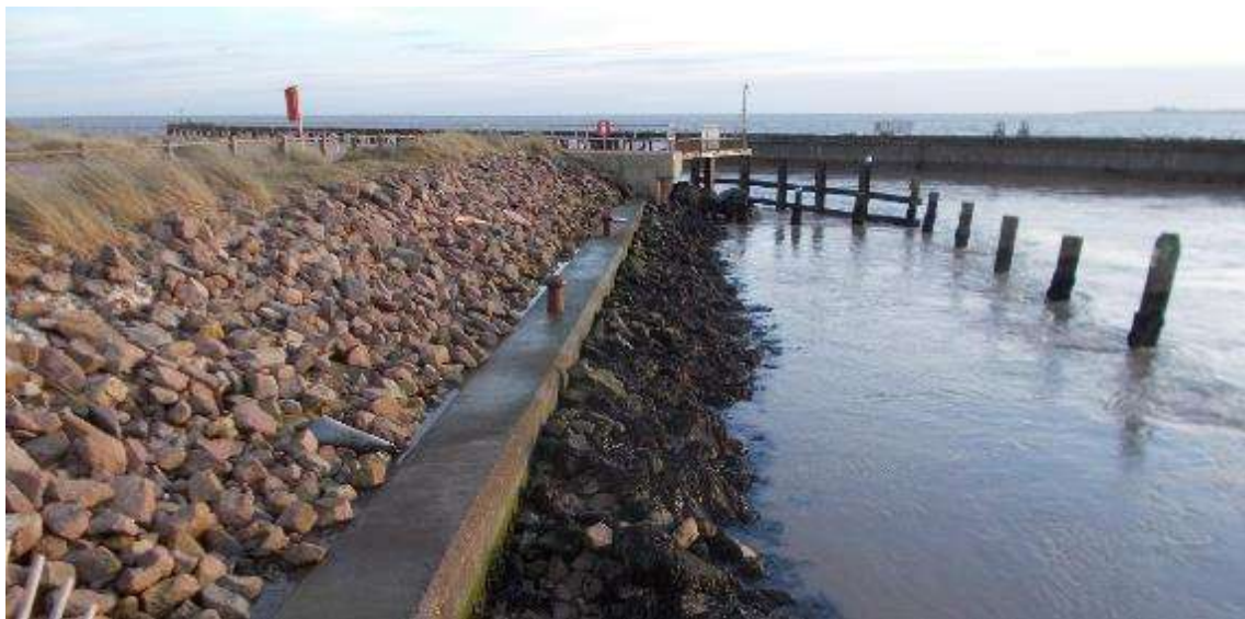
Figure 4-16: Current condition of Knuckle
