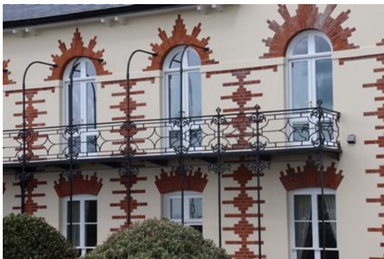
Restrained iron railings, supported below to form first floor balcony and covered ground floor veranda
