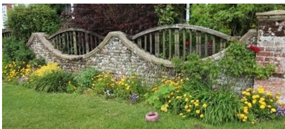
Cobble wall, stone caps and timber baluster screen to Commoners and Fairway Cottage, The Common
