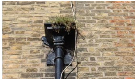
Good maintenance of this early 19th century rainwater hopper would help to prevent damp and damage to brickwork and other decorative features.
