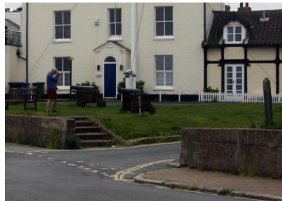
St James' Green: modern cement render (top) on earlier block wall and steps (below).
