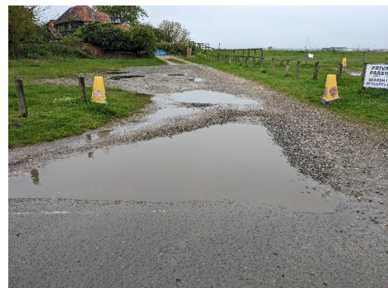
Figure 50 Signs of flooding at the time of survey (May 2023)
