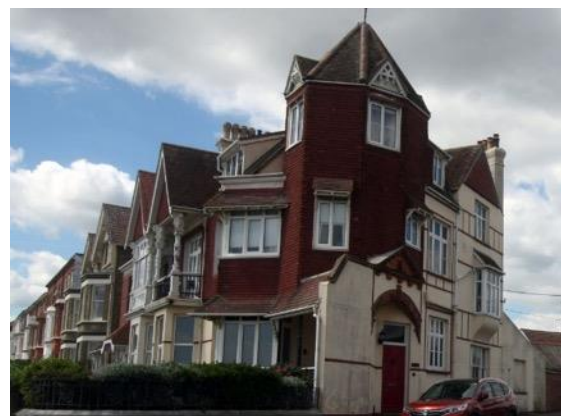
North Parade: some timber windows have been replaced with Upvc units at this prominent corner building.
