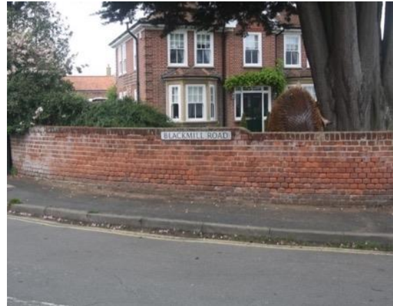
Blackmill Road (above): the effects of cementitious mortar pointing on historic boundary structures when combined with road grit and water spray from rain and passing vehicles.
