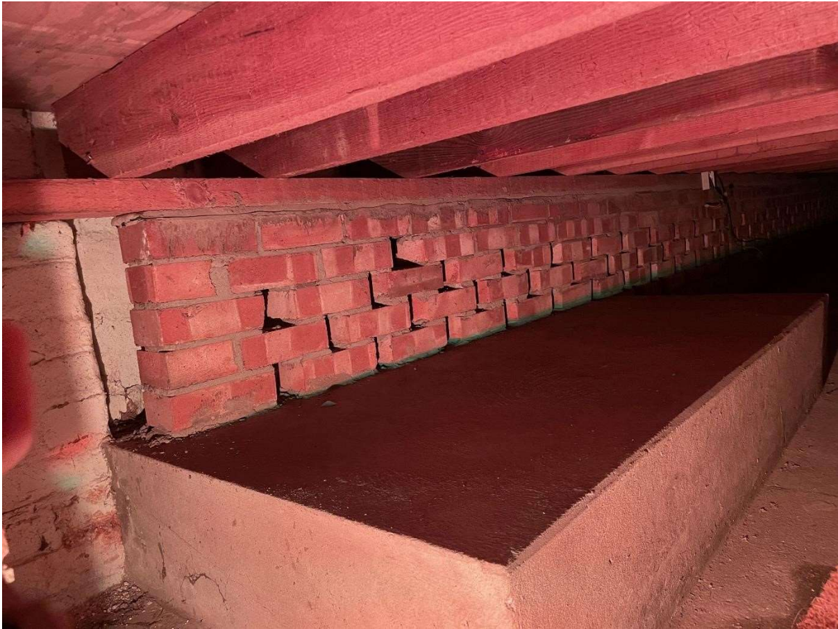
This is the space under the floor at the point of the proposed re-opening of the accessible entrance.
