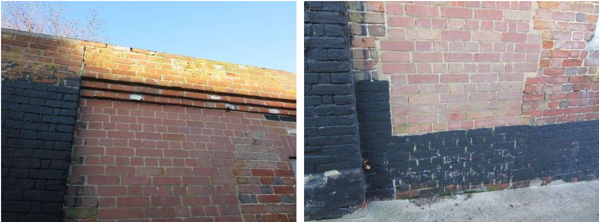
Proposed position for entrance door to warehouse. Evidence of a former opening here.
