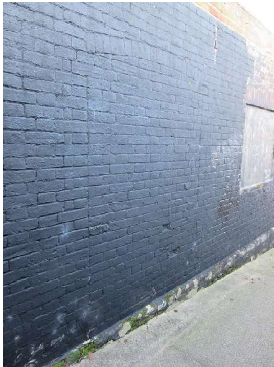
Proposed position for entrance doors to storage area. Evidence of a former opening here.
