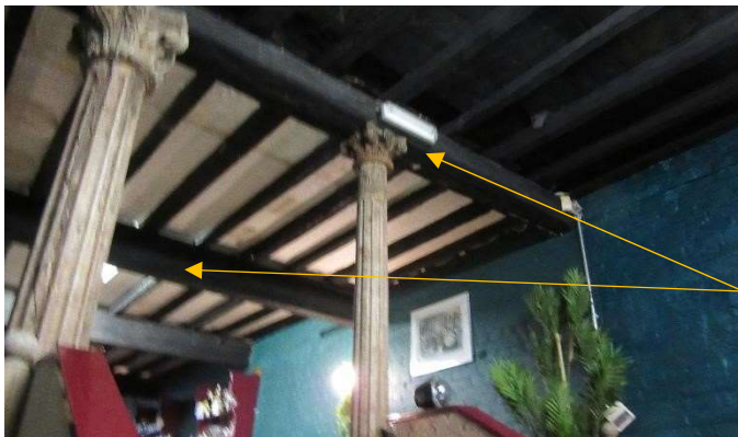
The partial replacement of the stud walls will be under these two existing beams. The pillars are temporary and only decorative.
