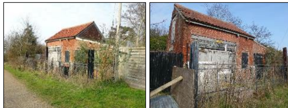
Figure 67: Vacant workshop/stable building along the footpath, that presents an opportunity for enhancement through maintenance works
