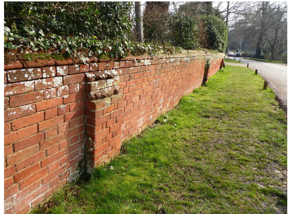
Figure 15: Red brick boundary walls within the Conservation Area are a key element (the location of important walls are identified on the map included in Appendix 1)
