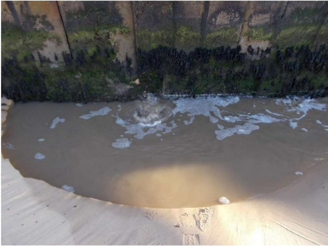
Figure 9 - Scour Hole in South beach at piles 66-67
