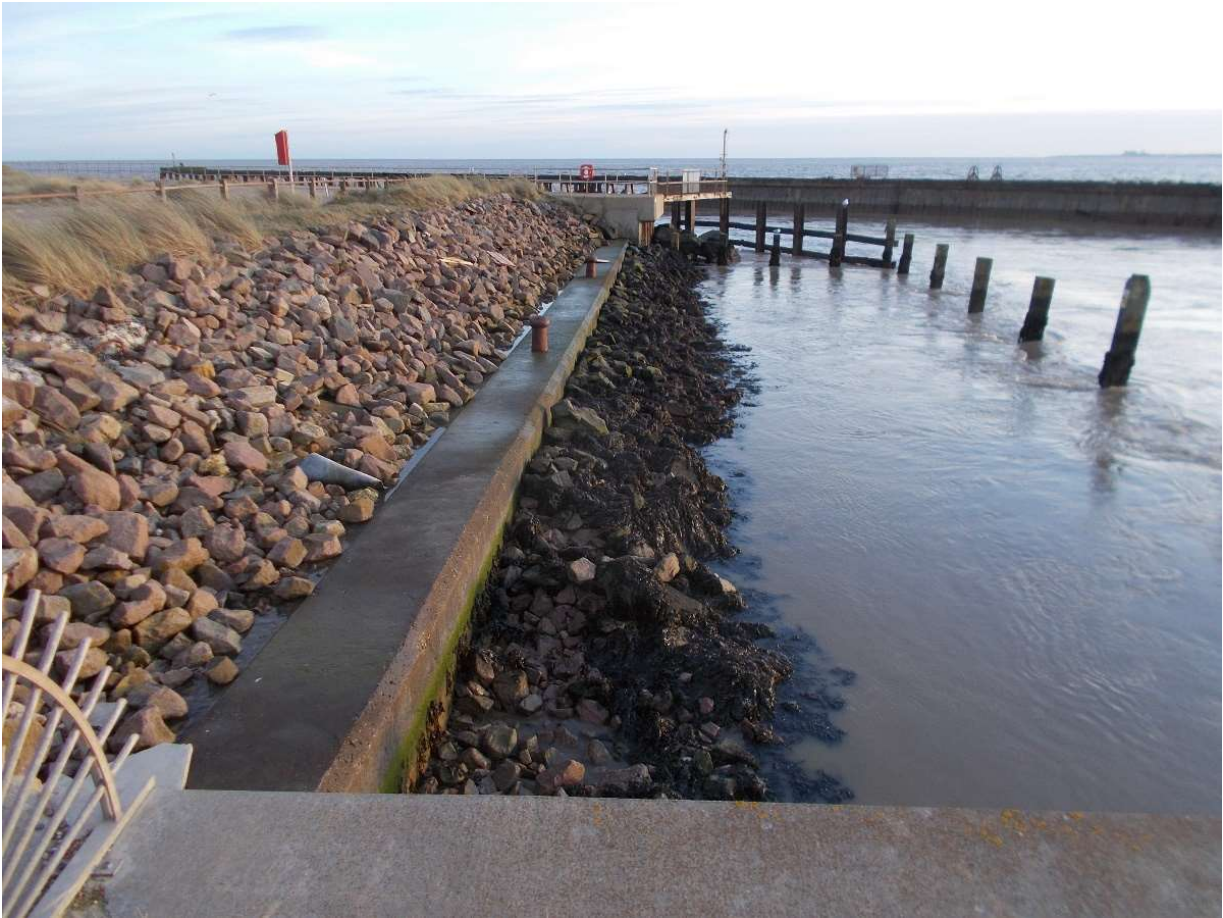
Figure 27 - Current condition of Knuckle
