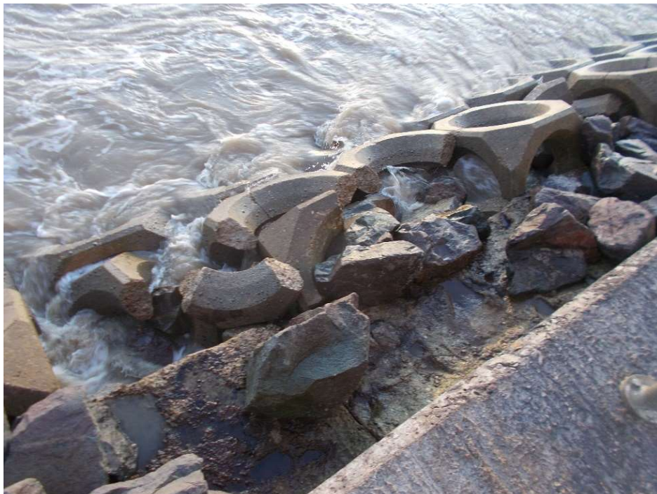
Figure 33 - Failed blocks near east end of concrete block revetment
