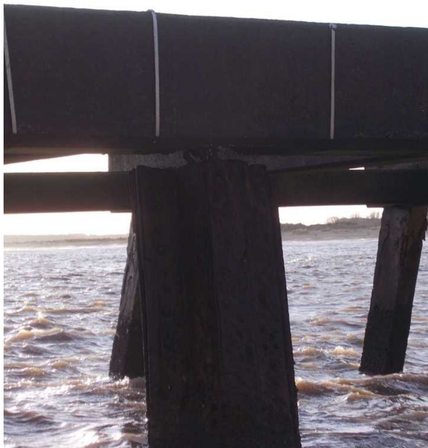
Figure 6 - Box Pile 8 failure
