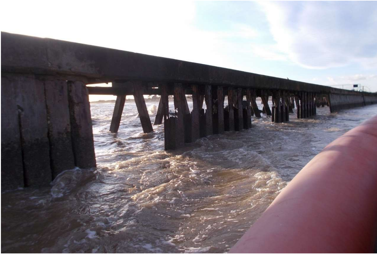
Figure 7 - Length C corroded steel sheet piles and unsupported front beam.
