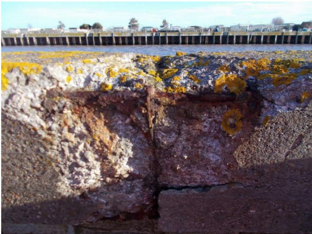
Figure 10 - Exposed rebar and failure of front beam at piles 115-116
