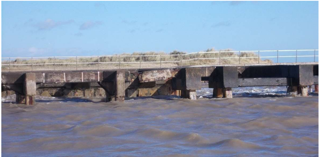
Figure 8 - 35-36 rear longitudinal beam failure
