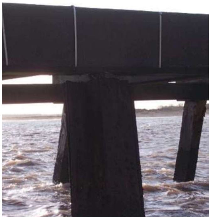
Figure 4-6: Box Pile 8 failure
