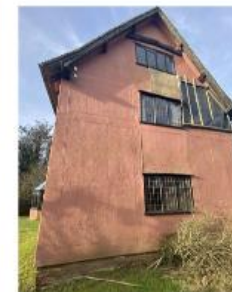
East gable showing temporary protection due to damage from recent storms
