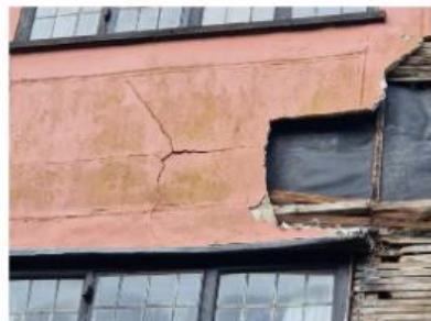
East gable highlighting exposed timber laths and damaged nails
