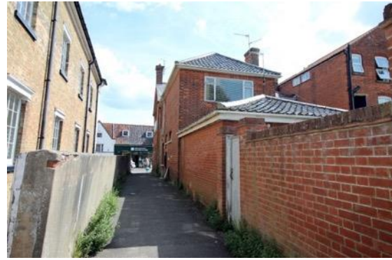
Woodleys Yard: This simple service lane has lost texture and visual interest with the use of modern cement render on an earlier brick wall. There is some evidence of damage to the brick as a result of water ingress.
