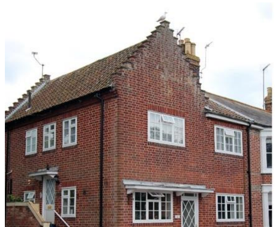
Variation in gable design across the Conservation Area makes a substantial contribution to the character and significance of the Conservation Area: Dutch and pedimented gable (top) and Crow-stepped gable (bottom)
