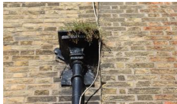
Good maintenance this early 19th century rainwater hopper would help to prevent damp and damage to brickwork and other decorative features.
