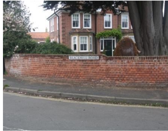
Blackmill Road (above): the effects of cementitious mortar pointing on historic boundary structures when combined with road grit and water spray from rain and passing vehicles.
