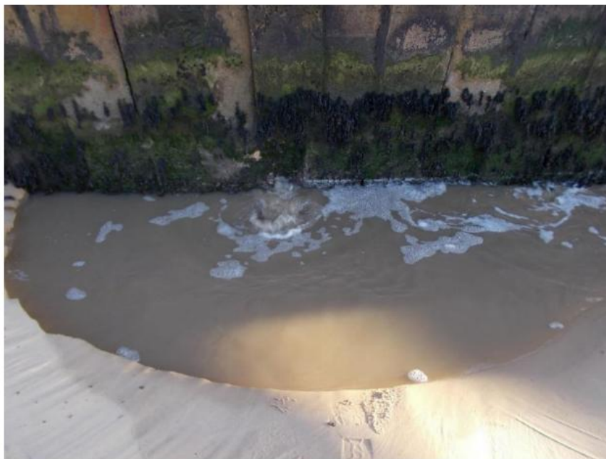
Figure 2-7 - Scour Hole in South beach at piles 66-67
