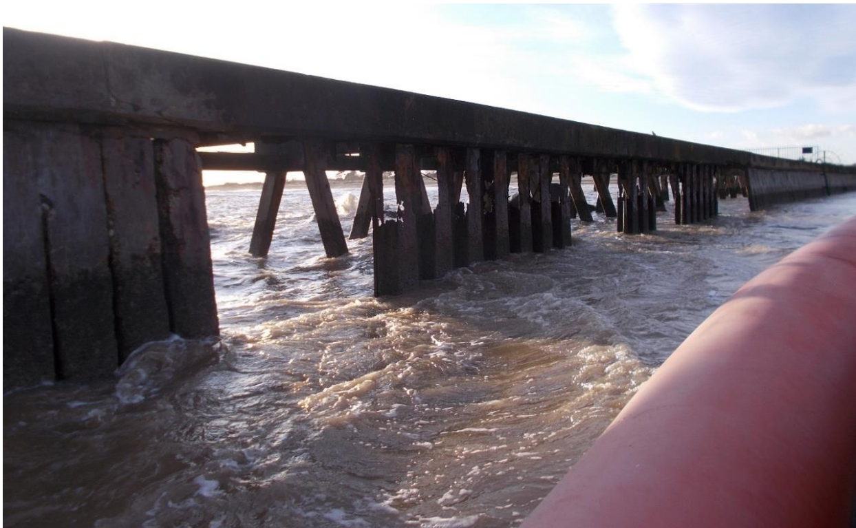
Figure 2-5 - Length C corroded steel sheet piles and unsupported front beam.
