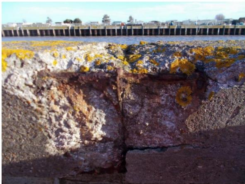
Figure 2-8 - Exposed rebar and failure of front beam at piles 115-116
