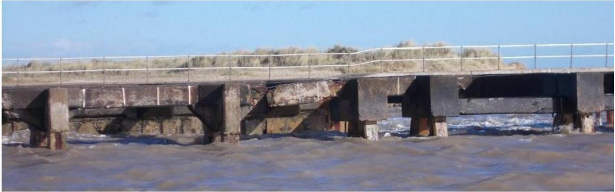
Figure 2-6 - 35-36 rear longitudinal beam failure
